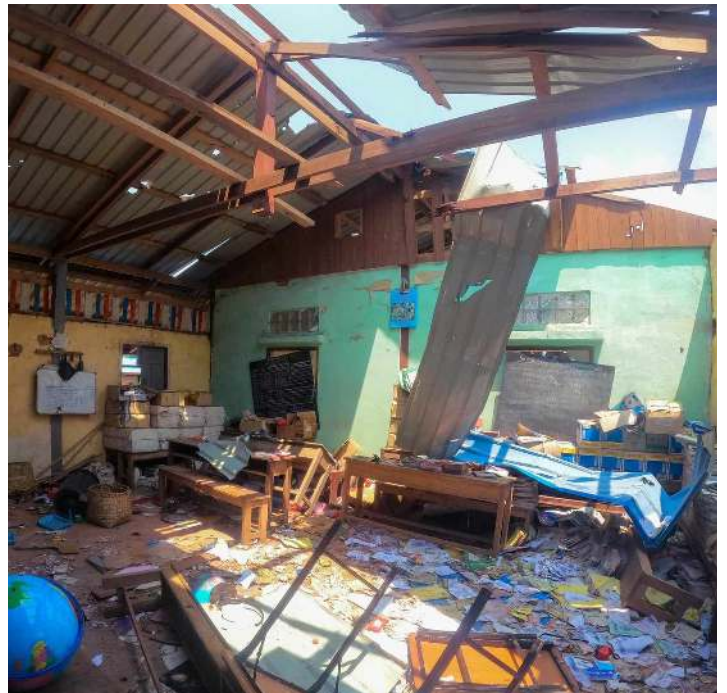
Community school destroyed by SAC air strikes, Mutraw district
